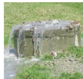
Sewerage overflow in their water catchment area.
